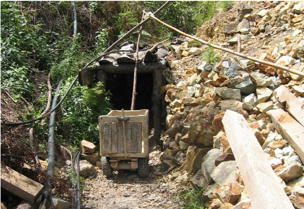
An Adit developed by artisan miners to the west of Hermans Find
